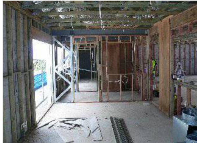
Looking through the media room, through the observation room, kitchenette and reception area, to the library entrance.
